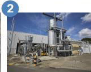
Biogas treatment plant
