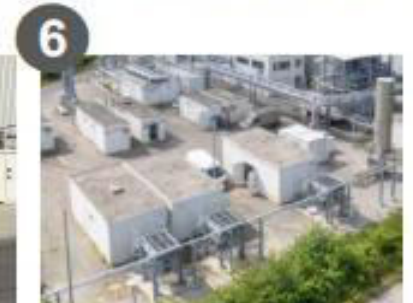
Hydrogen filling station
